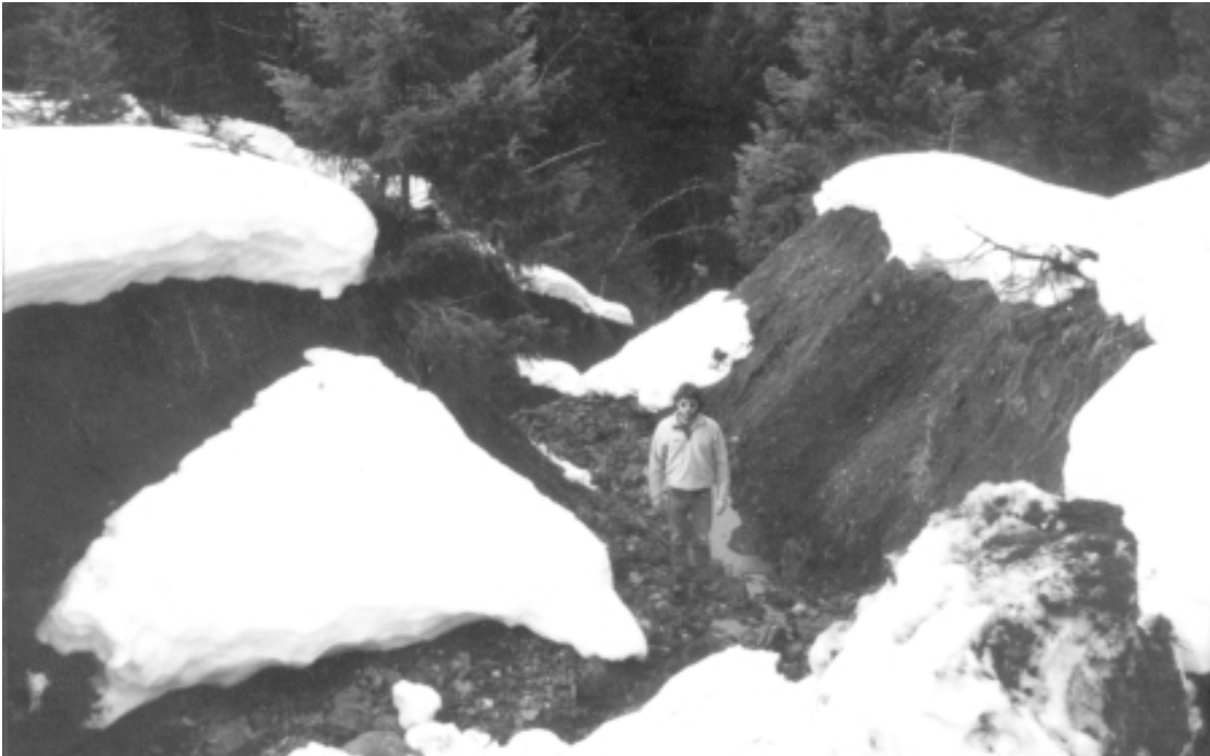
Figure 4—Diversions cause long-term gully erosion and damage to soil and watershed resources on both abandoned and maintained roads.
