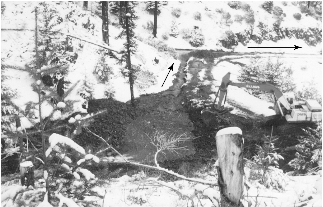
Figure 6—Cascading failure. Diverted flows from crossing A overwhelms crossing B, which also diverts to another crossing (not shown).
