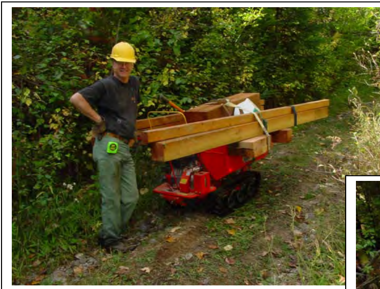
Trail Subcontractor transporting treated timber materials for construction of one of the trail puncheons
