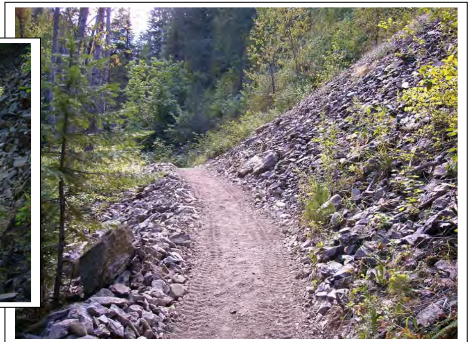
Trail construction through talus slope areas and placement of trail tread material
