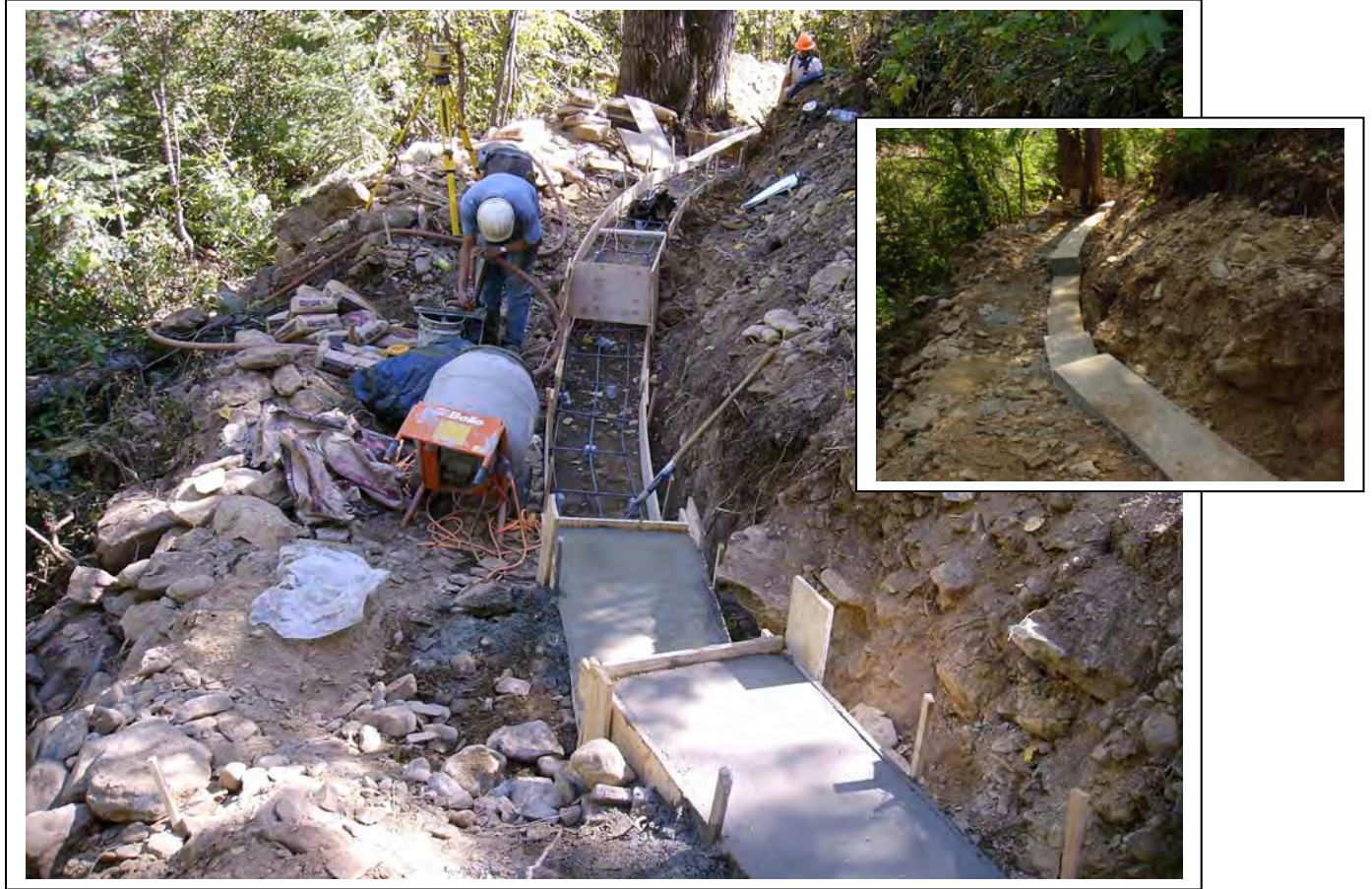
Concrete placement for modular block wall footing. (Note: new trail will be constructed on an elevated grade to the right side of photo)
