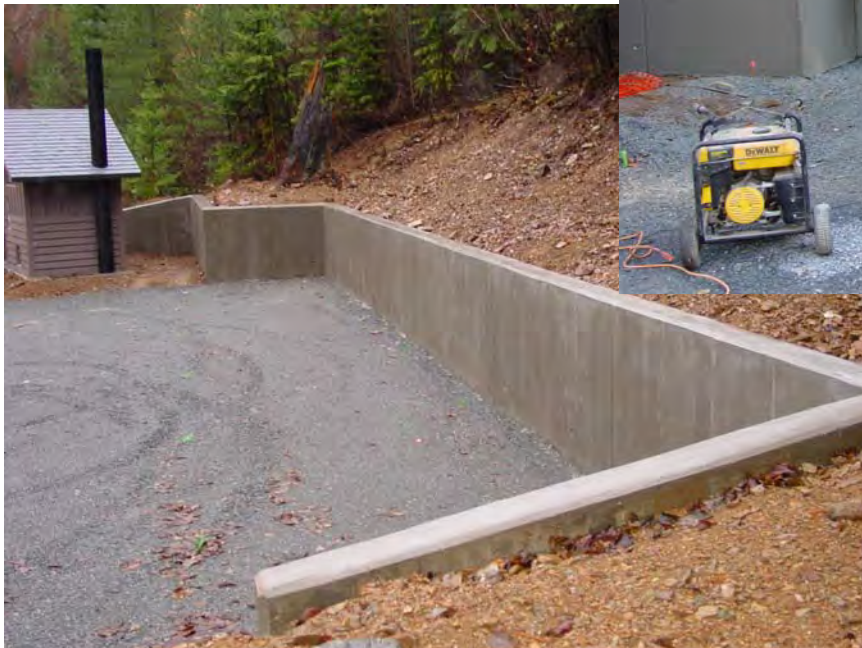
Finished appearance of concrete retaining wall after application and curing of Trammscrete product.
