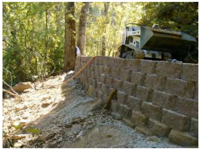
This section of completed modular wall will be over 7 foot high. At same location, the lower wall section is backfilled with embankment as illustrated in upper picture.
