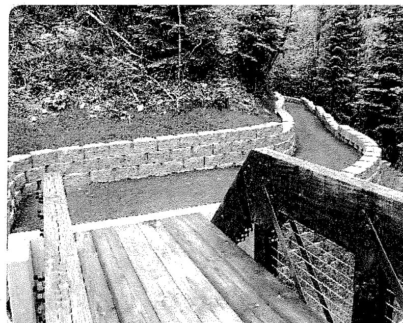
Coming off the ADA accessible Moosman Bridge onto the trail with MSE block walls.
