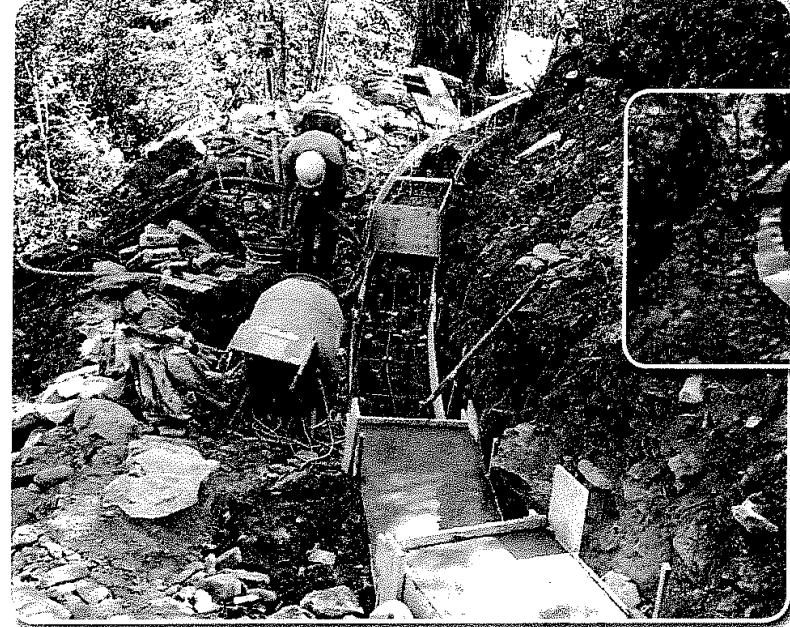
Poured concrete block, the use of the hand mixer was necessary because of the sensitive area.
