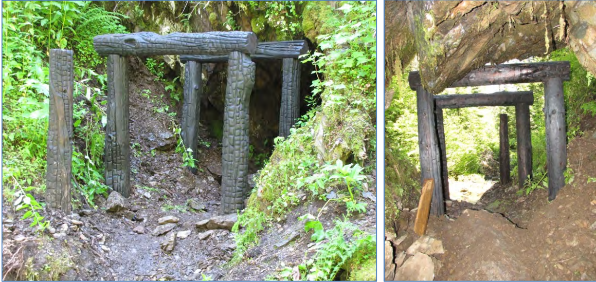
Figure 10. Finished portal reconstruction, viewed from both the exterior (left) and the interior (right) of the adit. Note the brace made of treated 2x4" lumber in the left photo. Each post had a horizontal foot nailed to the bottom that was set in a trench excavated perpendicular to the post. A brace was then nailed to the foot and the post to provide additional support. The braces were covered with soil if they were visible from outside. The braces on the left side as you look out of the portal were set toward the back of the adit, while the braces on the right side were faced toward the adjacent post of the same set (see Figure 7 right). The cap logs were placed in a saddle carved in the top of each post and drilled and fastened with rebar to secure them in place. A marine grade water proofing agent was used on the outside and cut ends of each log to reduce natural deterioration. It is expected that the structure will last about 10 years, which is pretty good considering sets in the Coeur d'Alene mines were generally replaced every three to five years.
