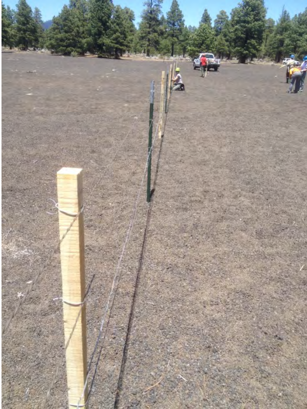
Figure 14. Enclosure fencing repair on May 23, 2013 at the astronaut training ground to prevent unauthorized motor vehicle use.
