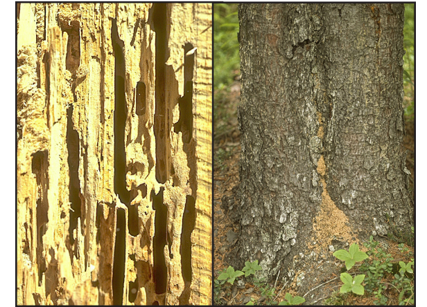
Figure 4. Left: Advanced carpenter ant damage. Right: Frass piles are evidence of carpenter ants. (Photos: Ed Holsten and Richard Warner, USDA Forest Service)
