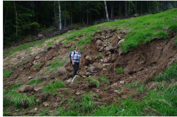
Single failed waterbar on newly constructed trail at Loon Mountain. WMNF photo by Joe Gill.
