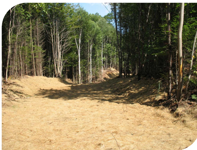
Straw mulch to prevent erosion and puddling. WMNF photo by Andy Colter
