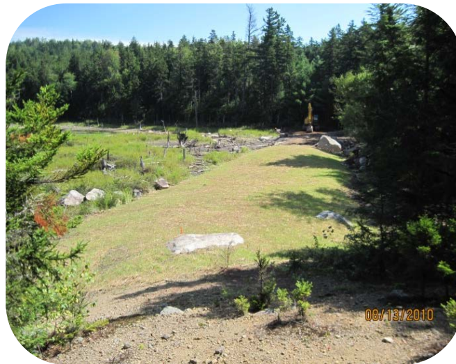
Completed work at the Province Pond dam. WMNF photo by Jacob Ormes.
