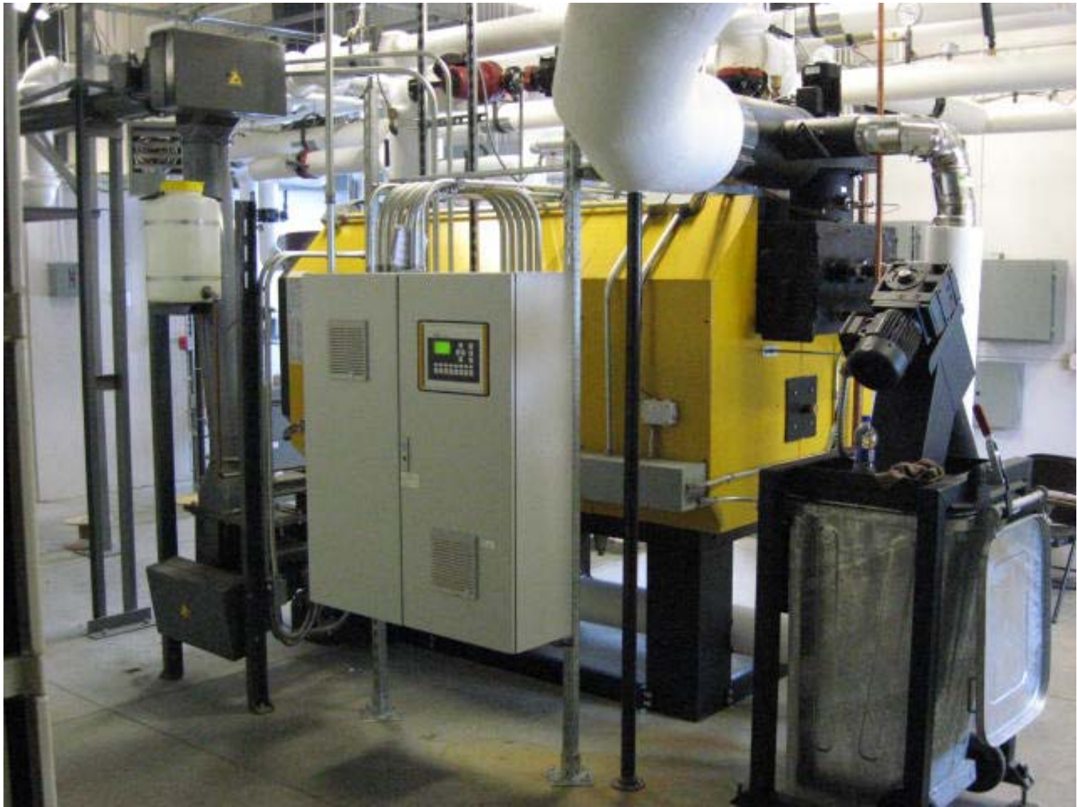
Automated Pellet Delivery and Ash Removal
