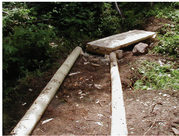
Tandem-packing bridge materials for Black Bear Bridge maintenance (top). Strawberry Creek, Continental Divide Trail turnpike construction (bottom).
