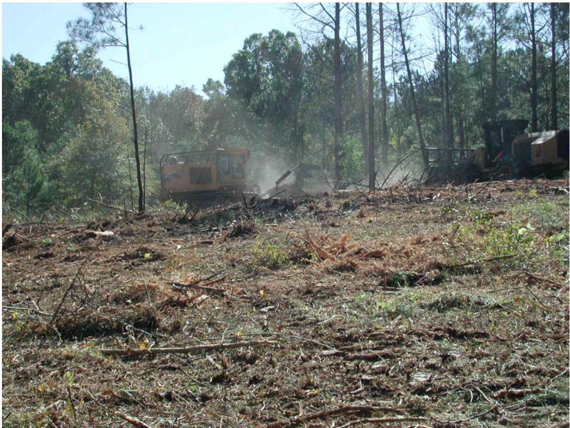
Cutting and grinding up of SPB killed trees on the Oconee Ranger District
