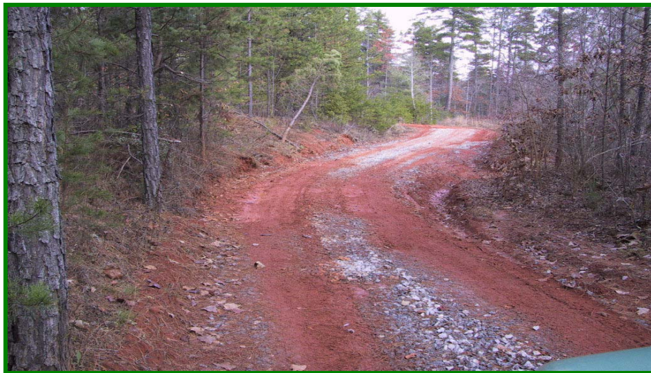
Figure 12 - Cross Drainage Culvert Needs to Be Install
