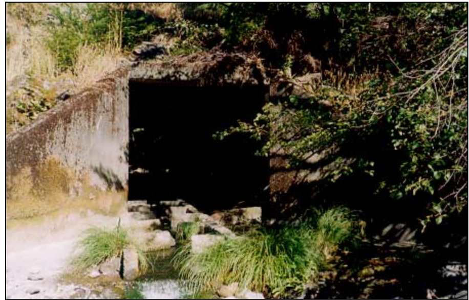
Figure 39. Cement culvert, with a fish passage structure, at the mouth of Williams Creek.
