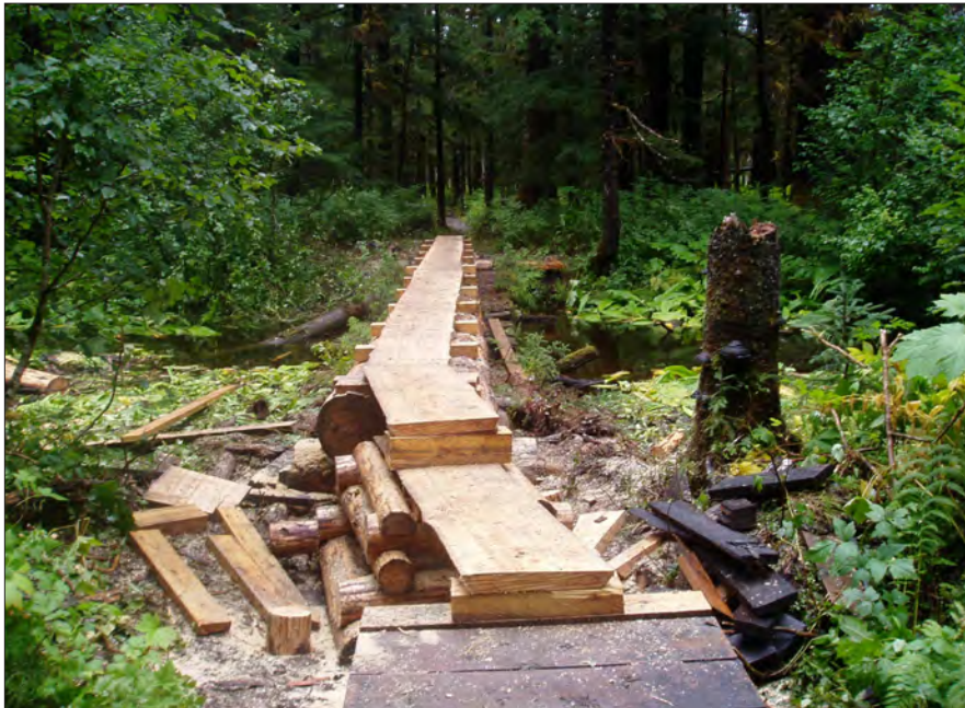
Work is underway to address a problematic section of the Windfall Lake trail. Photo by Peter Cross.
