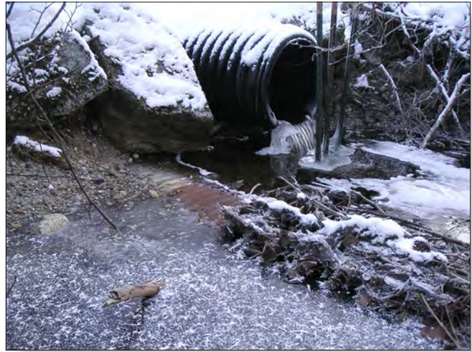
One section of a double culvert arrangement on the Dredge Lakes system is completely plugged.
