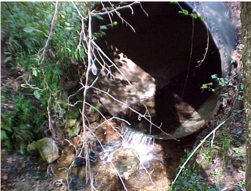
Figure 2. A culvert restricting fish passage.
