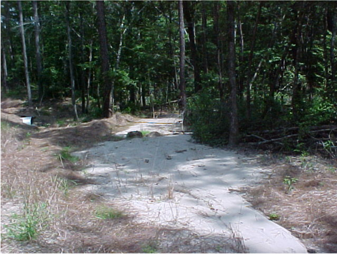
Figure 4. Wing ditch on new road depositing silt in riparian area and dumping directly into creek due to lack of J-hooking.
