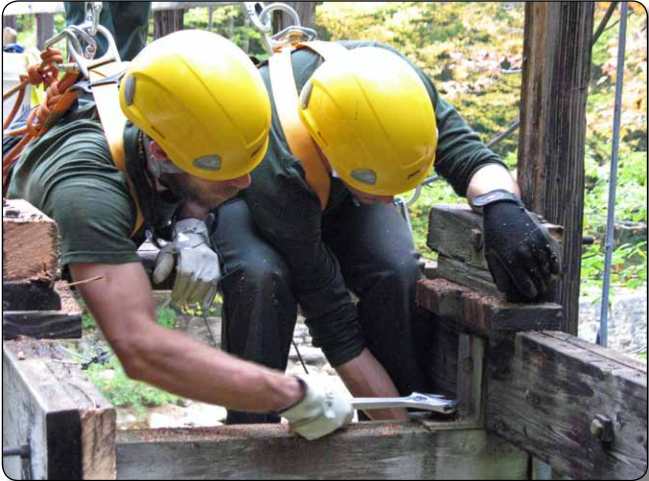
Figure 7. Forest Service employees dismantle old suspension bridge in the Pemigewasset Wilderness. WMNF photo by Tom Giles.
