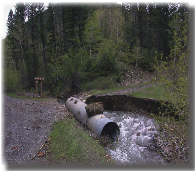
Washed out culvert, Helena National Forest
