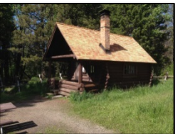
Spanish Creek cabin gets a new roof with the help of Gallatin Valley Backcountry Horsemen.
