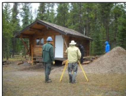
A Rendezvous Ski Trail warming hut cabin was installed during National Public Lands Day.
