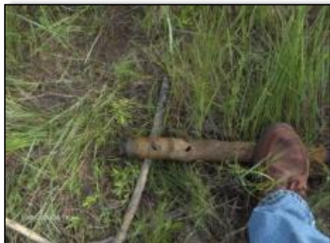
Holes in the old waterline at Buffalo Gap Campground were caused by a lightning strike.
