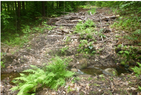
Skid trail crossing approx. one year after close out. Noted minor bank disturbance from placement and removal of bridge panels, which could be minimized by placing slash underneath before installing panels. WMNF photo by Sheila Johnson.
