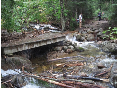
19-Mile Trail, damaged by Tropical Storm Irene. WMNF photo.
