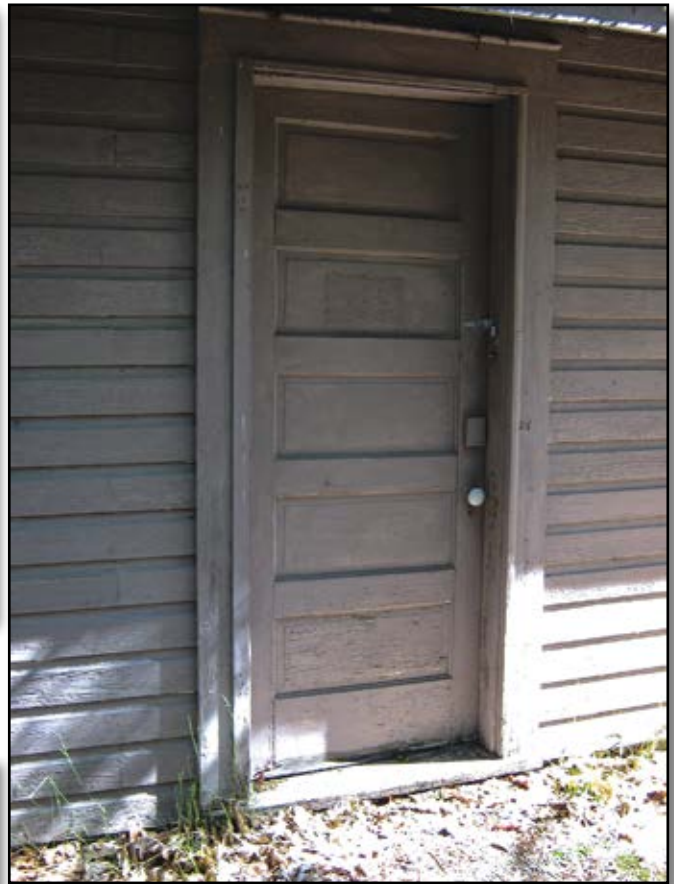
Figure 18—This rail and stile door is original to a mid-20th century recreation residence at the High Rollways tract of the Huron-Manistee National Forest in the Eastern Region.
