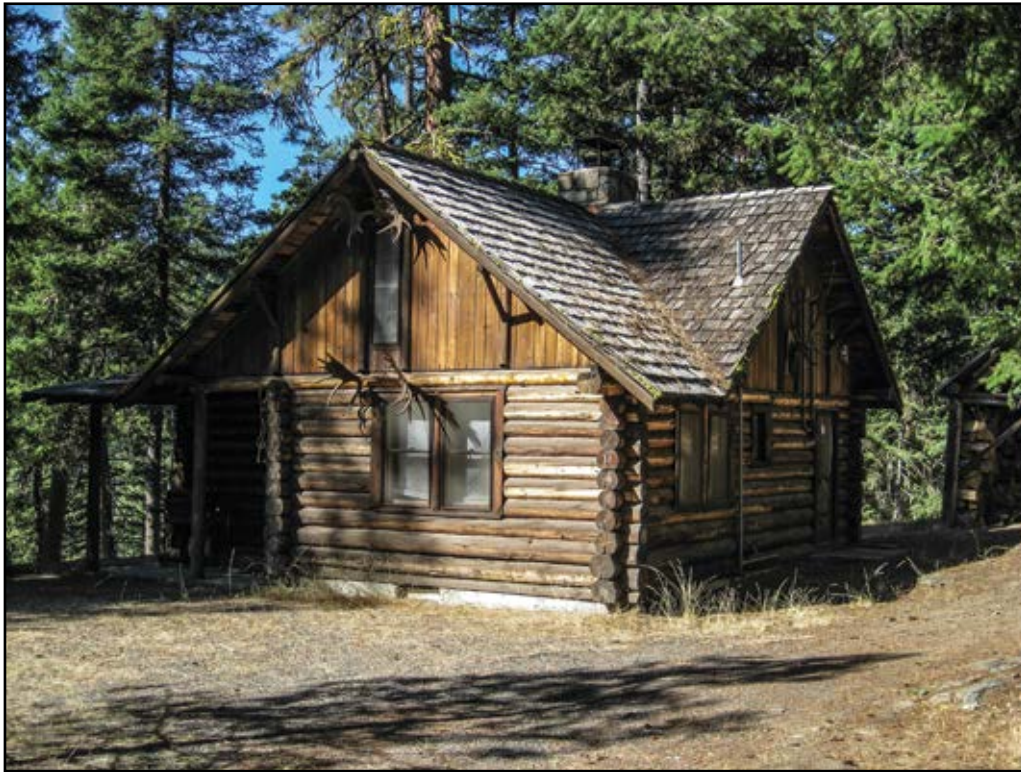
Figure 22—This 1948 recreation residence in the Hart Creek tract at the Okanogan-Wenatchee National Forest in the Pacific Northwest Region was built close to the ground on a concrete foundation. The low foundation has not led to deterioration of cabin logs because the climate is relatively dry and the soil drains well.
