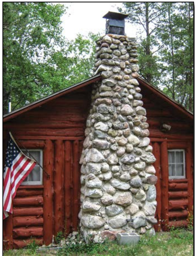
Figure 11—The fieldstone chimney extends well above the roof of this 1957 recreation residence at the Rollways tract of the Huron-Manistee National Forest in the Eastern Region. Smoke rises properly through this chimney that meets code requirements. A metal spark arrester prevents the escape of burning material that could ignite a forest fire.
