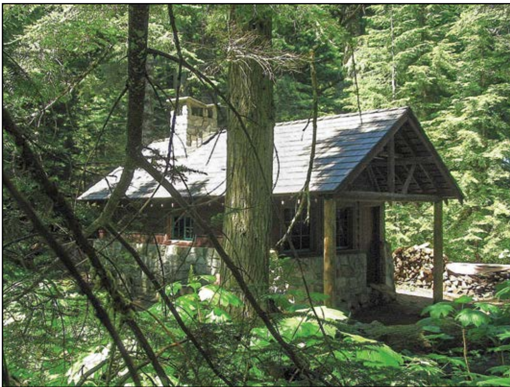
Figure 8—A tree fell during a storm and destroyed most of the original roof of this 1950 recreation residence at the Denny Creek tract of the Mt. Baker-Snoqualmie National Forest in the Pacific Northwest Region. The new roof structure and materials match the appearance of the historic roof, although the structure was strengthened to meet code requirements for snow loading.
