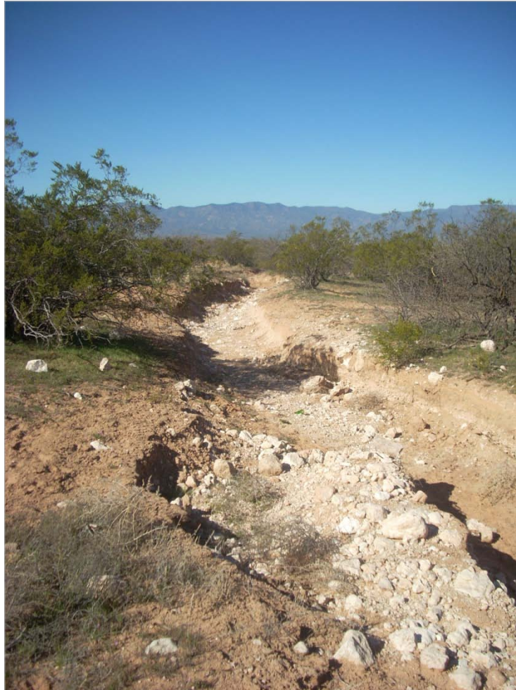
Figure 25. An unauthorized route in the Cornville area has become incised and acts as a channel to concentrate flows from rainfall
