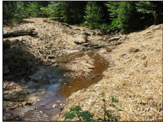
During the FR 182 decommissioning a culvert was removed to restore aquatic organism passage on Sugar Run.
