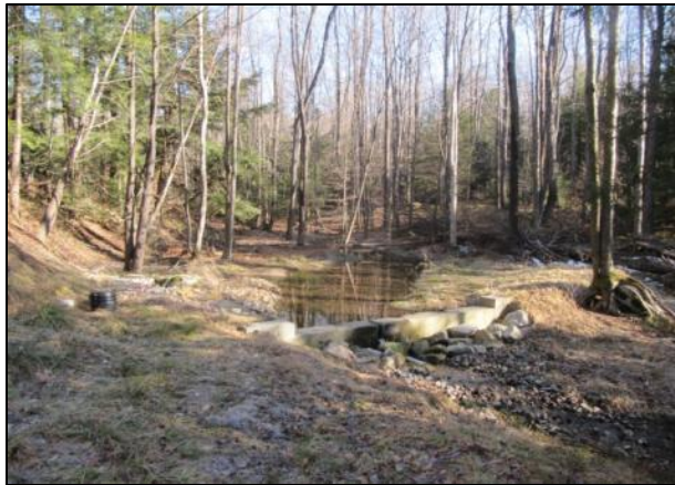
1 st - Water being diverted from the stream channel enters the treatment system through an intake pipe
