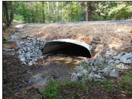
AFTER: A new bottomless culvert installed in 2012 to accommodate aquatic organism passage on Shingle Mill.
