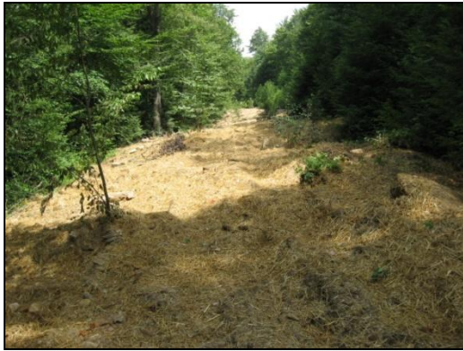
FR 182 has been re-contoured and planted with trees to fully decommission this road.
