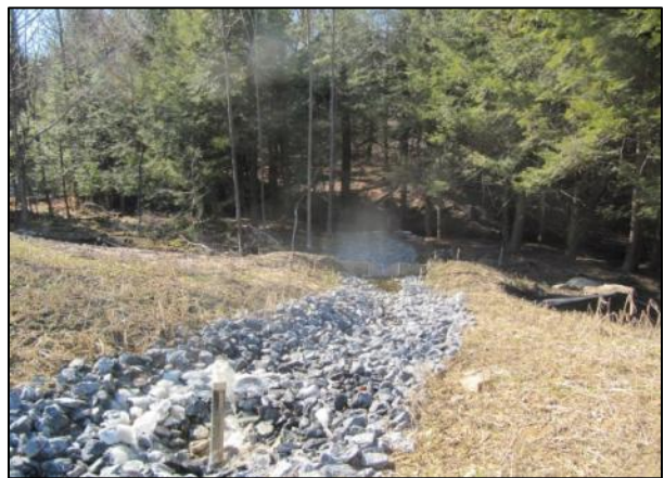
4 th - Treated flows back into the stream channel where the alkaline based water mixes with the calciteun treated acidic water, thus neutralizing the water that bypassed the system.
