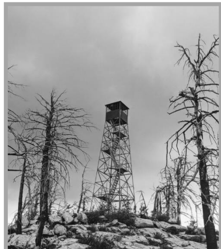
Figure 16. Webb Peak Lookout on Safford Ranger District was damaged by wildfire; a structural assessment has been completed and the Forest is exploring options to stabilize and repair the lookout, listed on the National Register of Historic Places. Photo courtesy of Maxwell Forton, USDA Forest Service.
