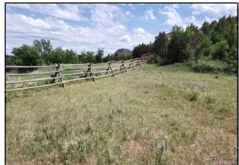
Recreation, Trails, and Fire staff work together to replace large sections of the buck and rail fence at the Magpie Campground.
