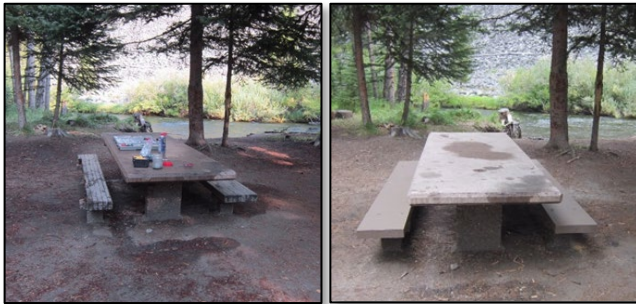
Before and after of benches replaced with lumber planks at Willow Creek Campground.
