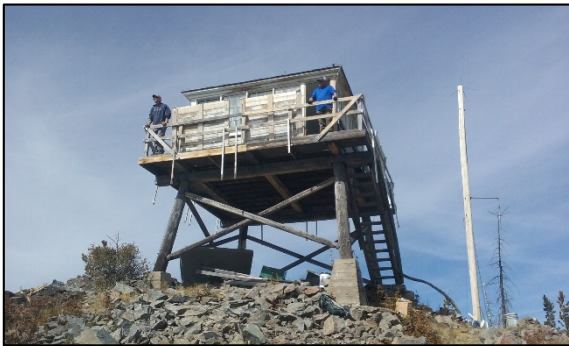
Recreation crew members prep Medicine Point Lookout for repairs and exterior and interior paint.
