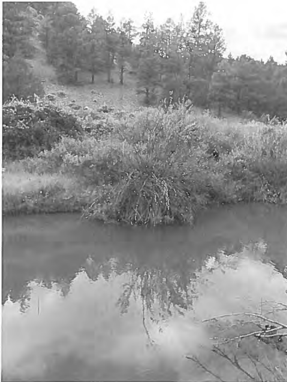
Over grown vegetaion on northside. North side needs lot of vegetation clearanc
