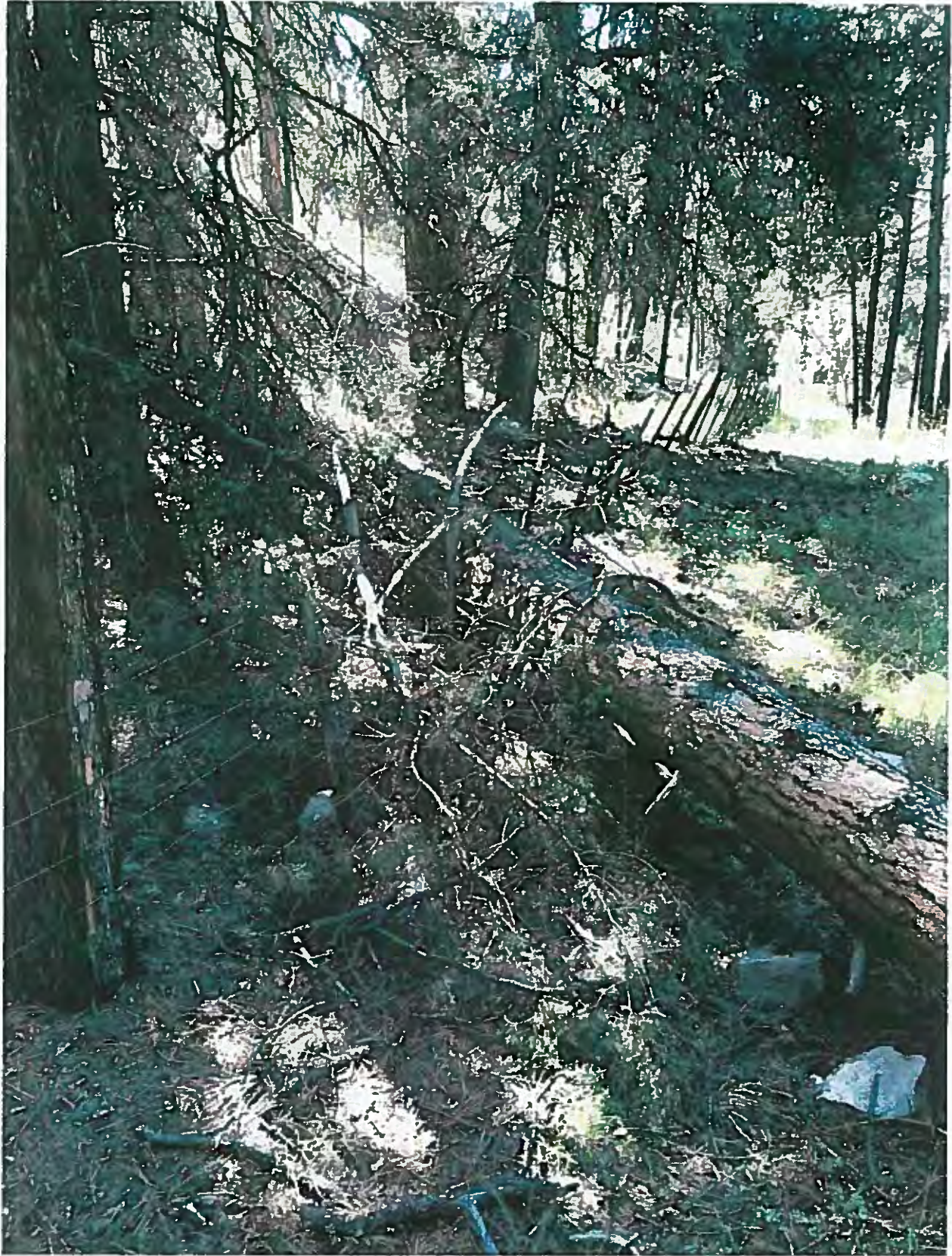
Figure 5 large panderosa pine damaging a section of fence
