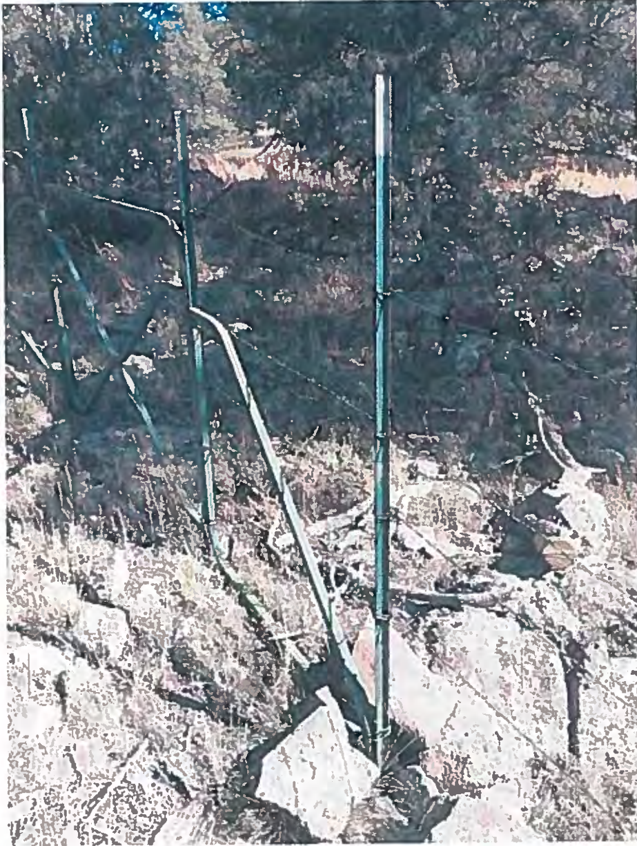
Dead branch on fence at corner fixed 9-2-2021
