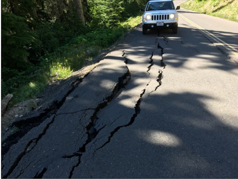
Photo 7. Example of road damage on a paved road
