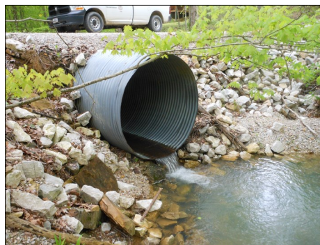
A barrier to fish passage in a stream.
