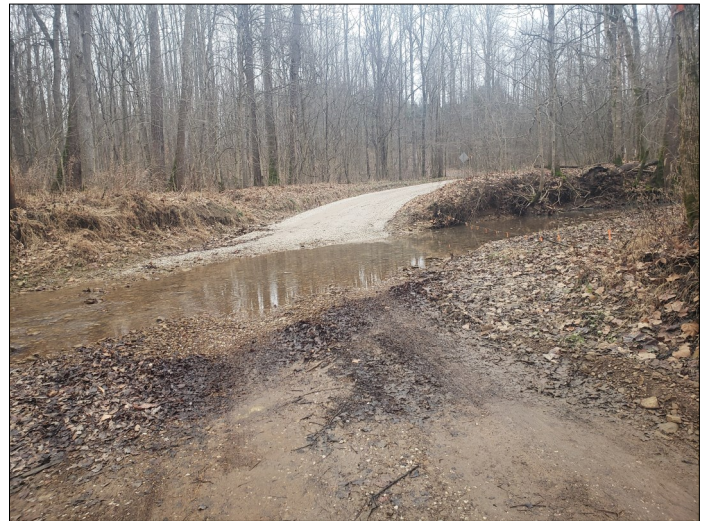
A county road crosses a stream which is a tributary of the Patoka River.
