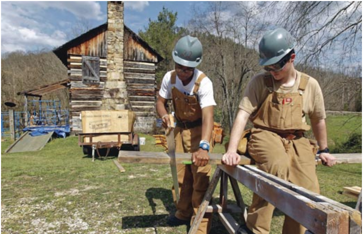
Frenchburg Job Corps students Demitri James, left, and Alex Fochtmann cut a board for scaffolding at the historic Gladie Cabin on the Daniel Boone National Forest in Kentucky. Job Corps students helped the U.S. Forest Service restore the historic cabin's shake shingle roof in 2013.
