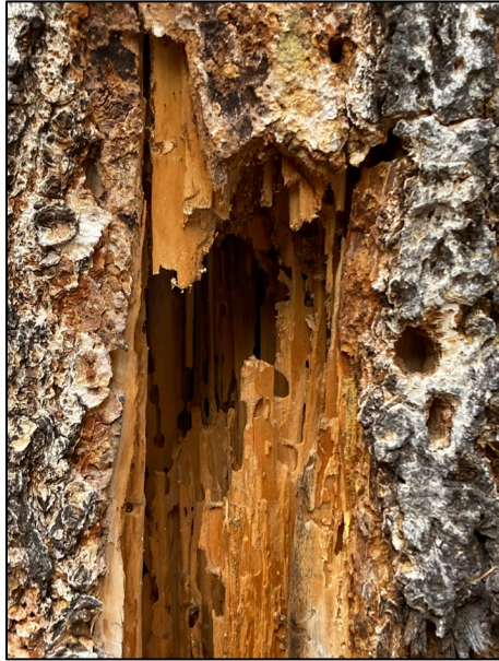
Figure 26. Carpenter ant damage.
