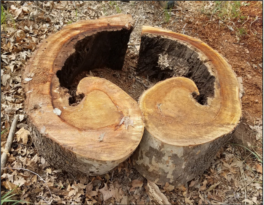
Figure 23. Ram’s horn crack from an Arizona sycamore.
