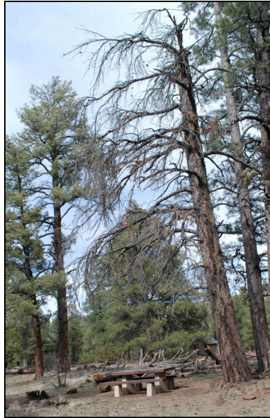
Figure 10. Failed top broken out of a ponderosa pine snag near high value picnic table and fire ring targets.
