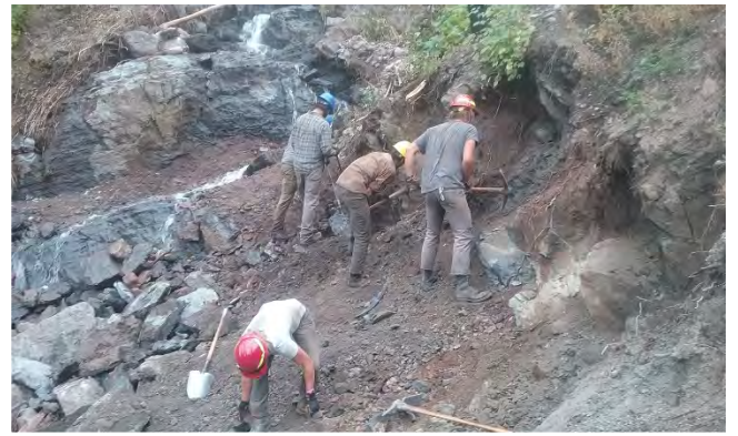
District Trail crew working on a blowout of Yellow Jacket Creek on the Monture Creek Trail #27. (2019)
