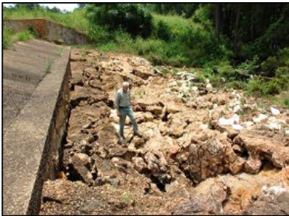
Ranger surveying damage to Ratcliff Lake Spillway. Erosion dropped the section he is standing on five feet.
