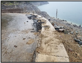
Boat launch before repairs
