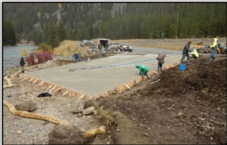
Contractors install the new concrete boat ramp at Moose Creek Day Use
