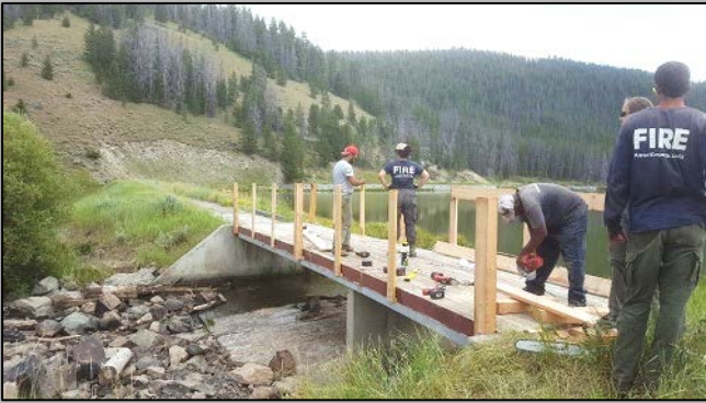
AmeriCorps crew at work on an accessible bridge located at Maney Lake.
