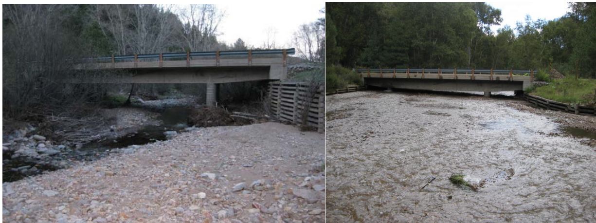
Figure 54. Bridge 107C in 2009 (left) and in 2013, one year after the Little Bear Fire
