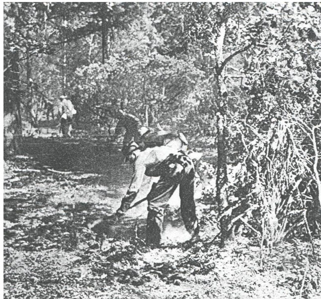
Building fire line
