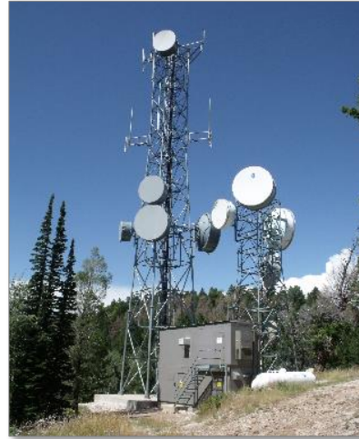
Communication site atop a ridge in the Ashley National Forest
