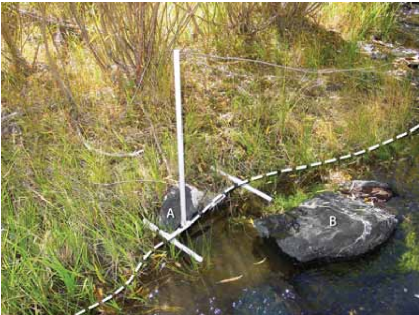
Figure A20. Rock "A" is embedded and above the scour line. Active erosion exists on the streambank side of rock "B," and it is below the scour line.
