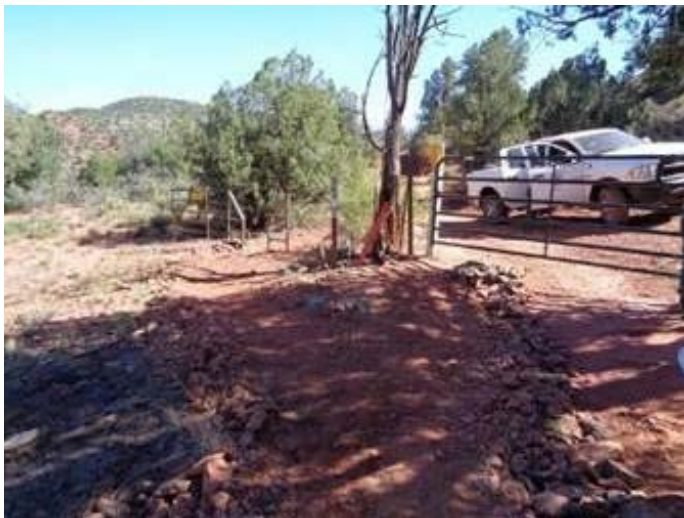
Figure 3. Gate installation included installation of a foot-travel and equestrian pass through, as well as erosion control features to restore gullies in the road.
