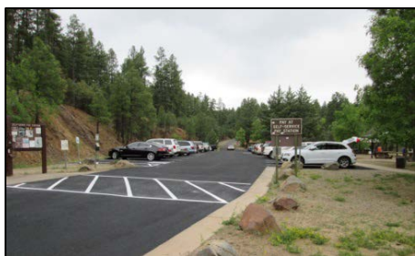
South Shore Boat Ramp and Picnic Area after seal coat and re-striping.
