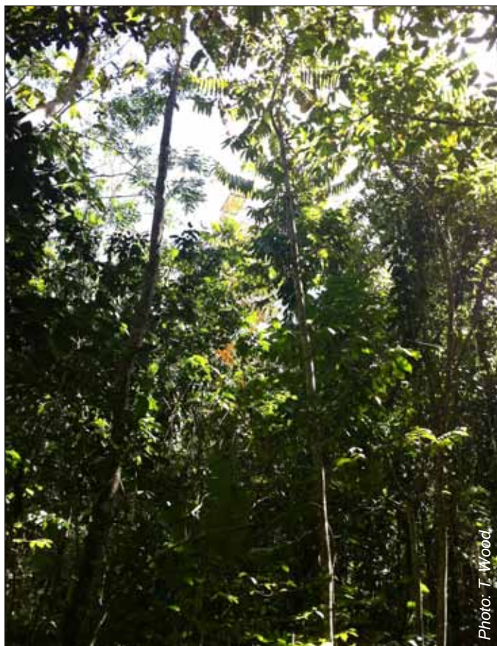
Two solar panels were installed above the forest canopy on existing towers to power an automated soil respiration system (Li-Cor LI-8100/8150) in karst forest at El Tallonal.
