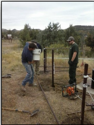
Recreation, Trails, and Fire work together to install a fence around the Coal Creek Campground solar well.
