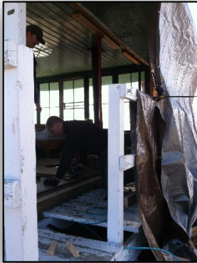
The forest partnered with the Northwest Montana Forest Fire Lookout Association to rebuild two walls of the historic Sex Peak Lookout.
