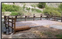
The fishing pier at Spring Gulch was repaired after damage from a pine tree.
