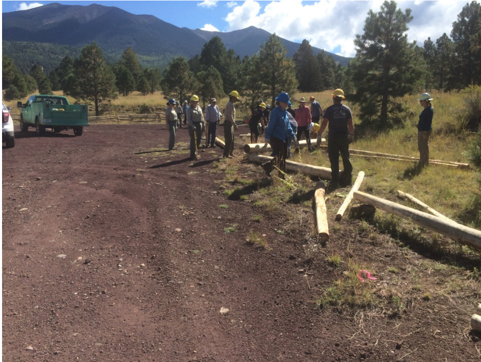
Figure 1. Installation of a log pole fence around the parking area at 9007T
