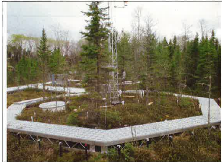
Boardwalk constructed at Spruce Site. Photo taken in May of 2014. Open air chambers will be constructed around these boardwalks and a variety of experiments will occur inside the chambers.
